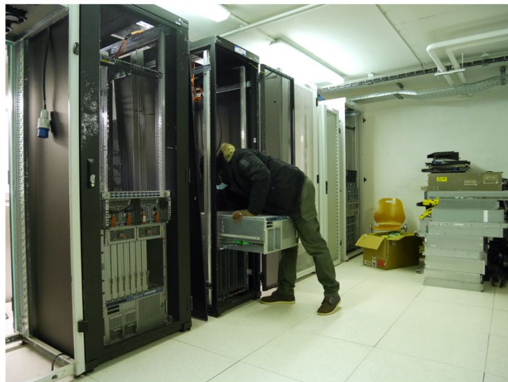
Salle technique (ici racking)
